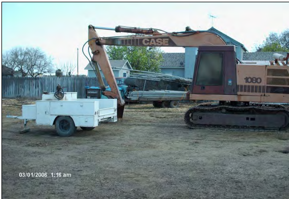
Figure 6-13. View Looking South of Excavator and Trailer with Fuel Pump & Tank (APN 047-025-022)
