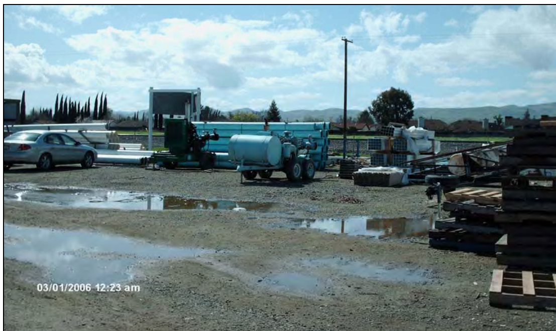
Figure 6-11. View Looking West of Mobile Water Pump and Tank (APN 047-031-039)
