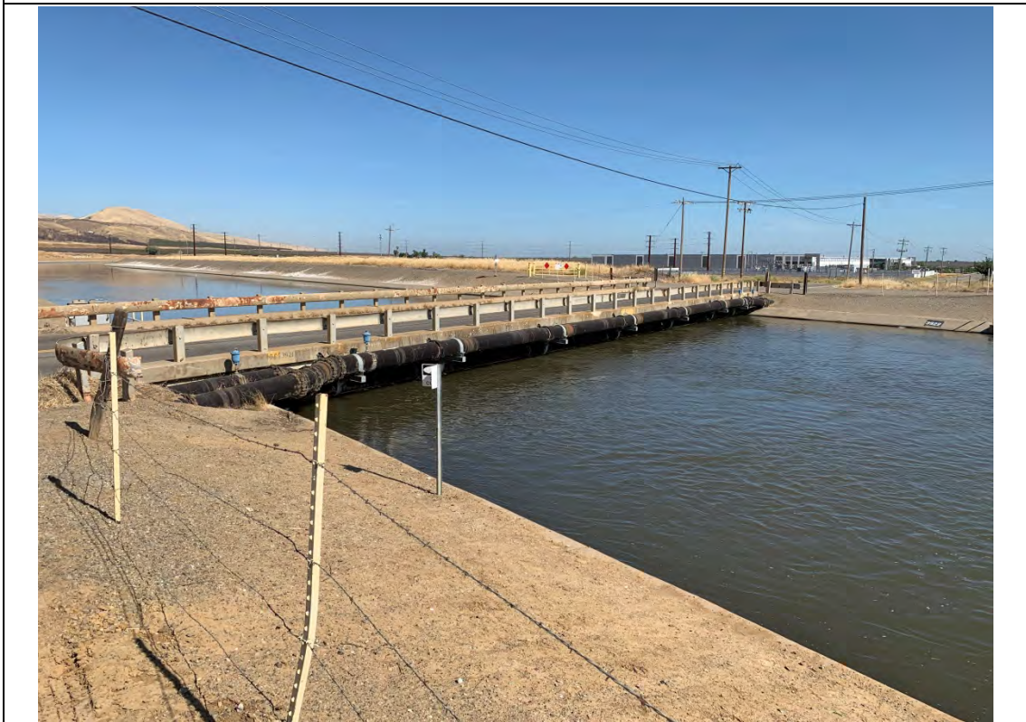
View of the Rogers Road Bridge over the Delta-Mendota Canal, facing northwest.
