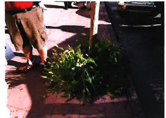
Weeds and cracked sidewalks were seen on S. Del Puerto Avenue.
